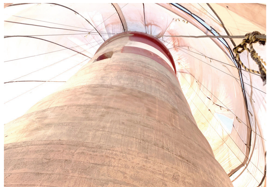
► The last section of paint that was stripped off under the tarp. KENT LEBOUTILLIER
